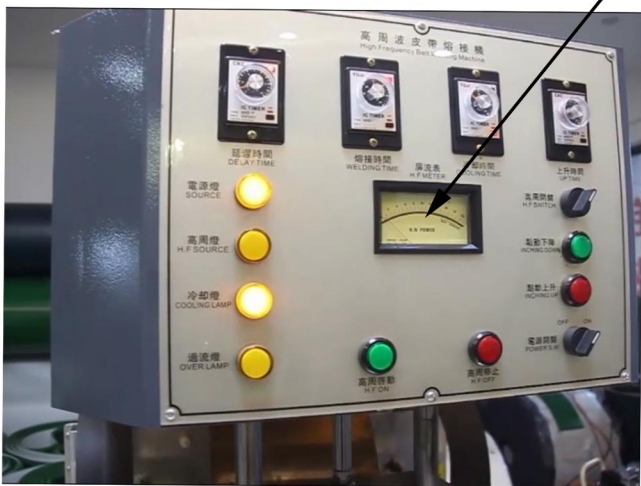
14.Check this part,you can see the H.F power.
